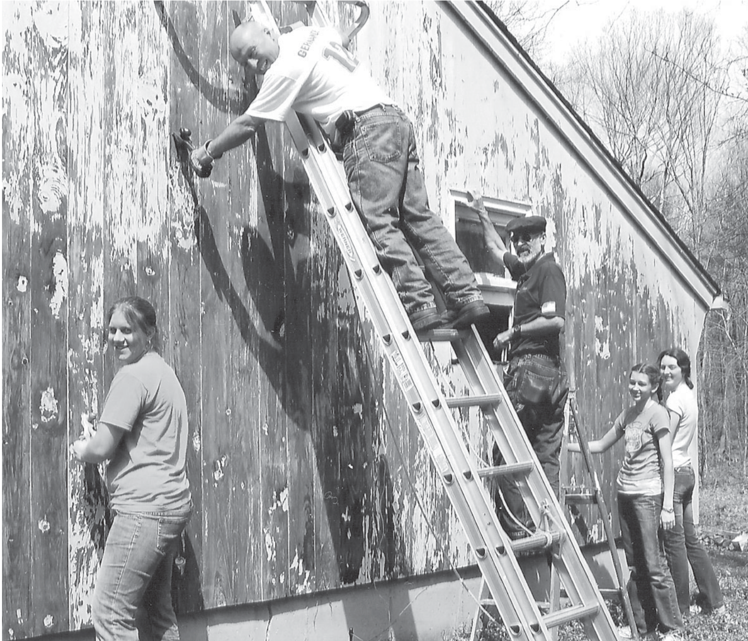
Victoria Boshart, Norm Dorval, Mickey Groshart, Rachel Mathiau and Katie Czaja (l-r) work together to paint a building during last Saturday's Helping Hands project. The Hebron Lions and RHAM Leos teamed up to assist six needy families in their spring cleaning.
