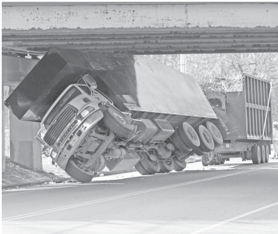
Didn't Quite Fit... This was the scene Tuesday morning on Route 2 in Marlborough, when the driver of a tree removal truck left his boom up and got stuck under an overpass, causing the vehicle to tip on its side. No injuries were sustained and the bridge suffered only cosmetic damage, according to the state Department of Transportation. A full story on this incident appears on page 24.
