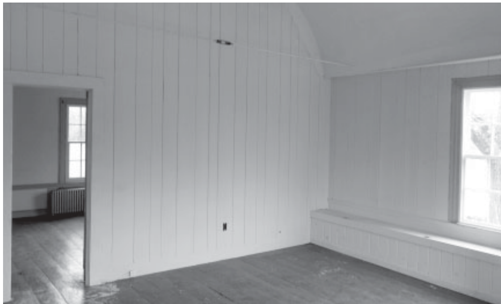
Inside the Peters House, volunteers are needed for all kinds of interior renovation work including the demolition of some modern changes – like the partition that was placed in the middle of the ballroom, shown here.
