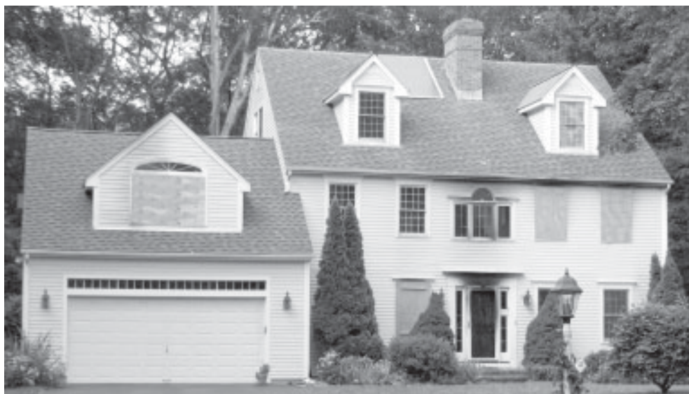
The fire that damaged the home at 64 North Maple St. was extinguished within an hour in the early morning on Thursday Aug. 8. The photo above was taken Tuesday, Aug. 13, and shows the aftermath of the fire that left the house indefinitely uninhabitable.
