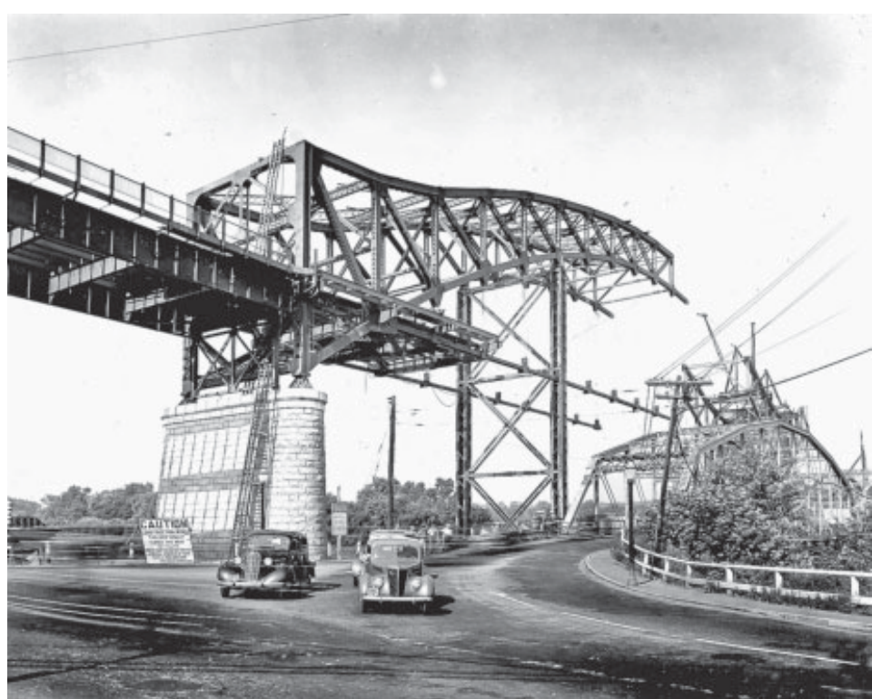
A Glimpse of Portland Past... This photo, taken during construction of the new Middletown-Portland (later rededicated as Charles J. Arrigoni) Bridge in 1936-38, shows several cars coming off the 1896 bridge on the Middletown side of the river. The old bridge remained in service throughout construction. The picture is one of many featured in the "Portland River Crossings" exhibit, which will be open this Sunday at the Ruth Callander House Museum of Portland History. For more information, see a related story on page 22.
