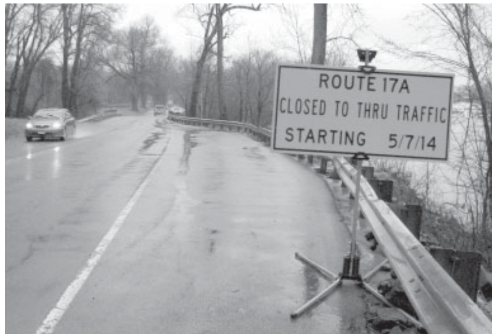
The Carr Brook portion of Route 17A will be close Wednesday, May 7, through Oct. 1 for roadwork and bridge replacement.
