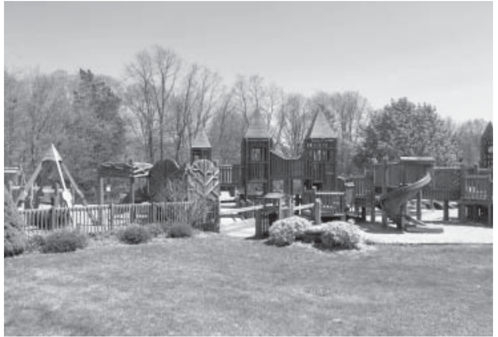
Some upset has been expressed recently over the Seamster Park playground near Memorial School, which is facing demolition next spring due to safety concerns.
