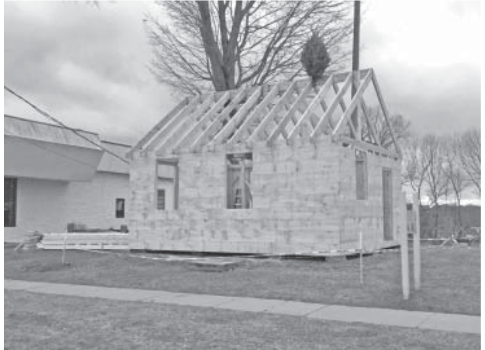
Construction of the ‘new’ School for Colored Children building is expected to be completed in mid-March and will be donated to the town as a gift from members of the Liverant family.
