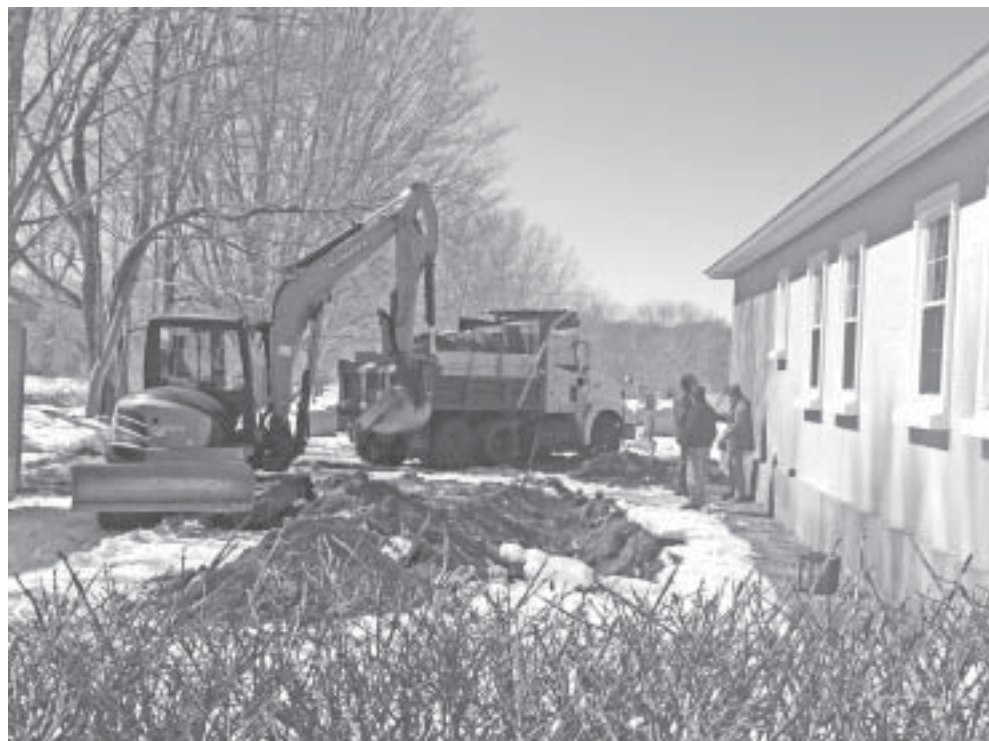
Workers gather on a chilly Wednesday at the construction site for the expansion of Phelps Hall at St. Peter's Episcopal Church.
