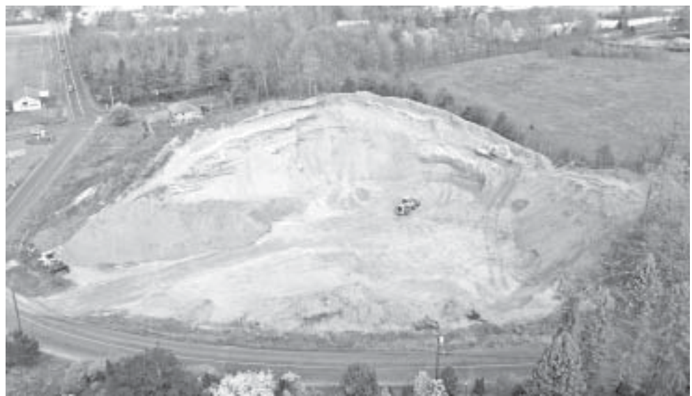
An April 30 aerial view of selectman Ben Srb's property on the corner of Sage Hollow Road and Cornwall Street shows the extent of excavation being conducted in accordance with a zoning permit for a single-family home. The town's current zoning guidelines allow the work to proceed unregulated for five years. Photo by MetroDrone LLC.
