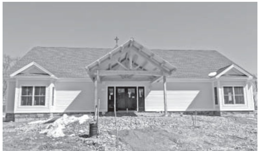
Work on The Worship Center's new sanctuary and ministry building, located at 99 Marjorie Circle in Hebron, is nearing completion – in the hopes the first services will be held there in July.
