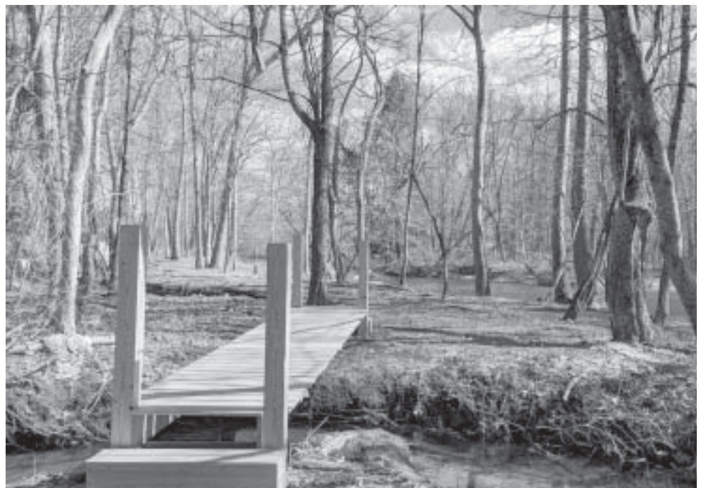
Scott Person, his son Justin Person and Planning and Zoning Commission Chairman Eric Anderson built this bridge on a flood-prone area near the Hop River behind Andover.
