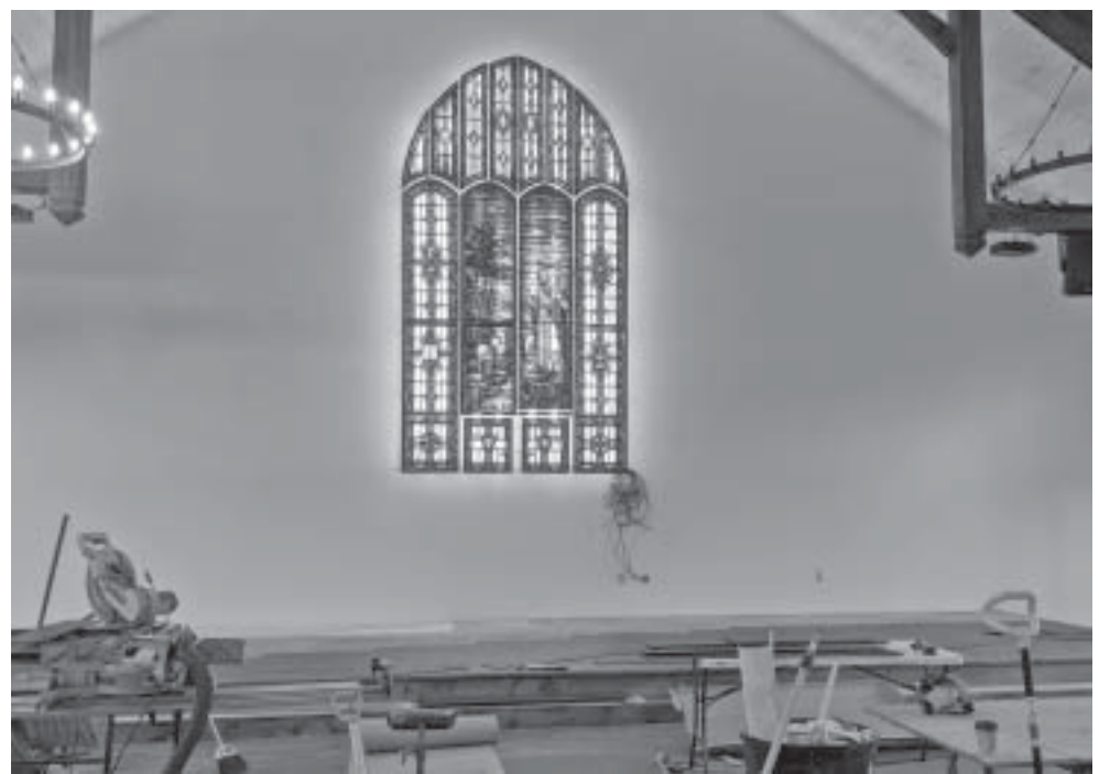
A 14-by-10 foot backlit stained glass window depicting the Good Shepherd is the focal point of the nearly-completed new Worship Center building. Plans are for the first service to be held before Thanksgiving.
