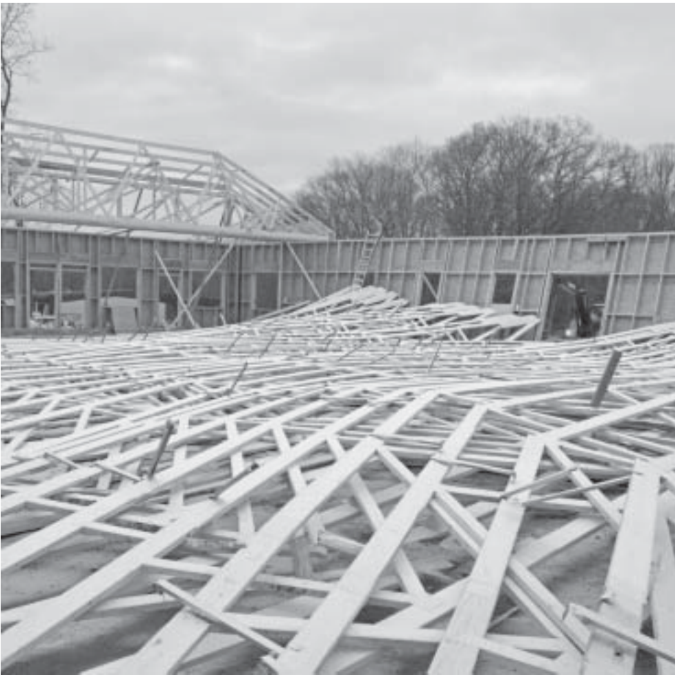
Officials said a Jan. 17 construction collapse on West High Street in East Hampton left three workers injured after approximately 20 roof trusses, each 74 feet long, fell "like dominoes" into the structure. Photo credit: East Hampton Building Department
