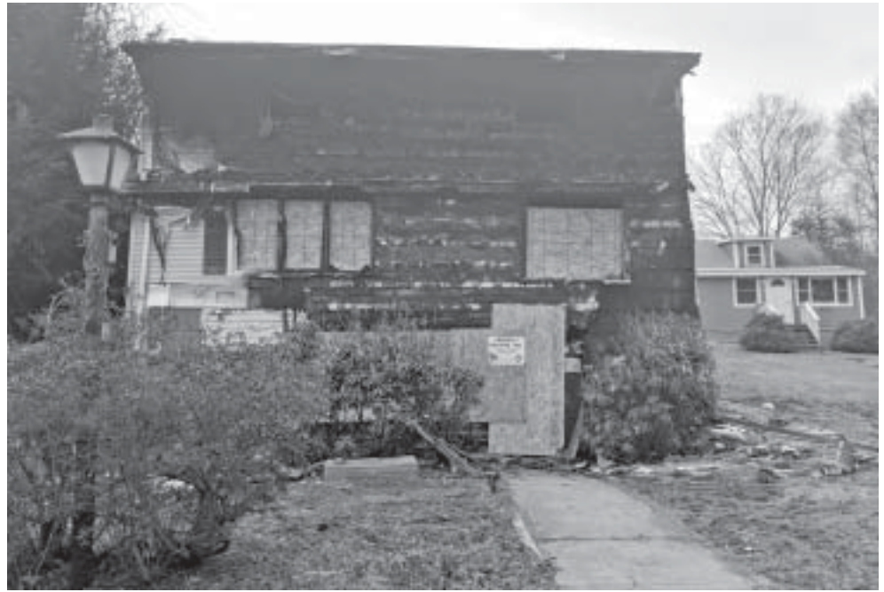
The house at 165 Lake Road was heavily damaged by fire on Dec. 21. Residents of Andover and surrounding towns have donated truckloads of items to the family that lived there with a month-old infant.
