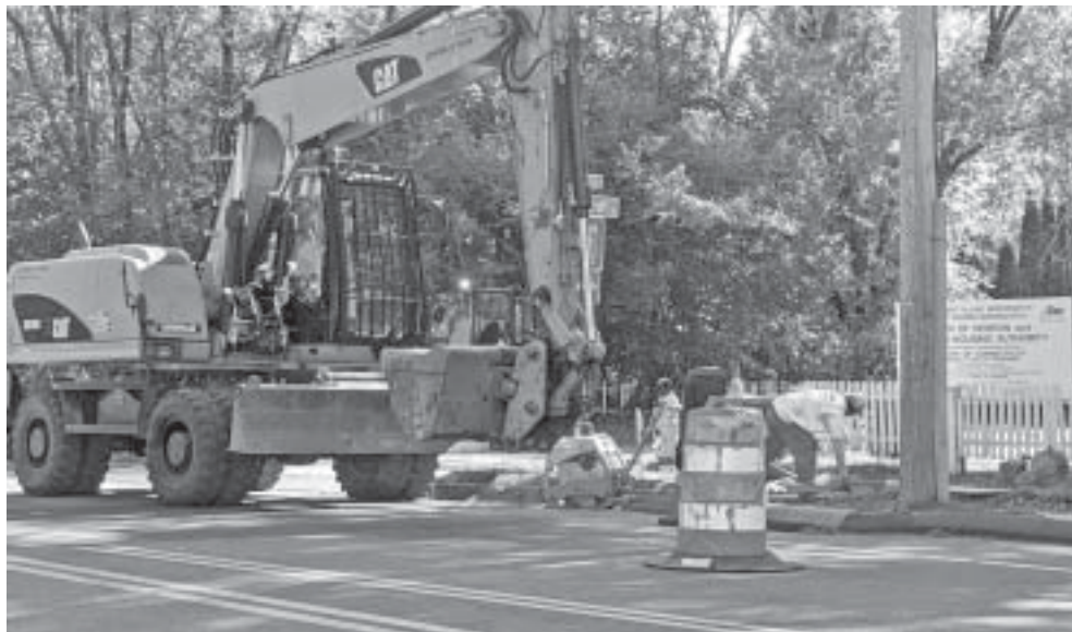
Sidewalks being installed on Church Street in Hebron will increase the connectivity in town, which is part of the town's long-term plan and, among other things, will make it easier for seniors to walk from Stonecroft Village to the center of town.
