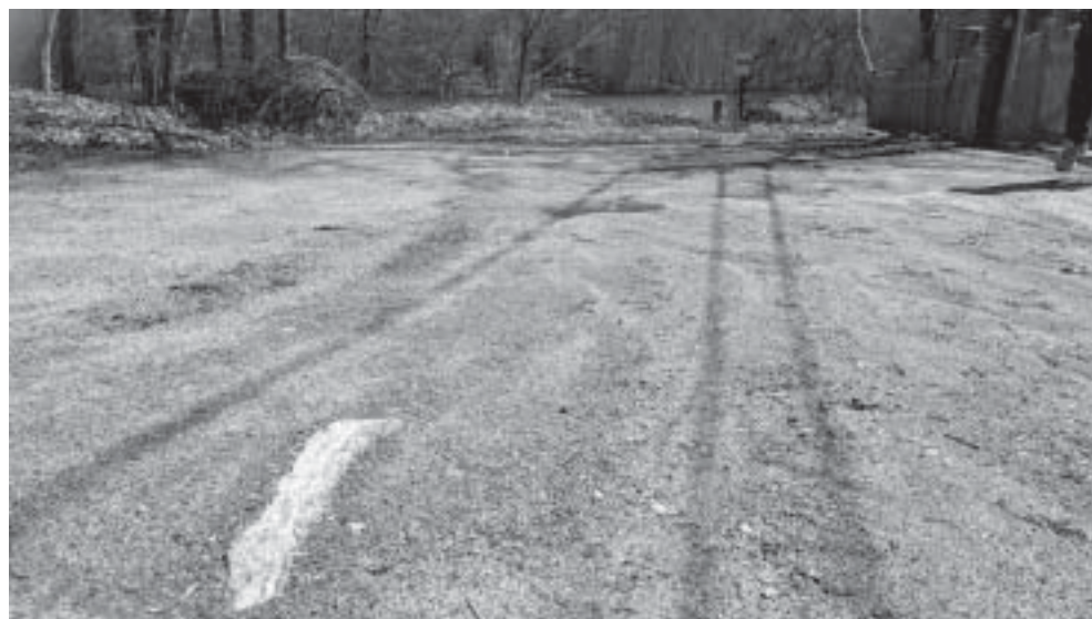
Sunset Lane, a short dirt road off Lakeside Drive, is on a list of roads that need to be paved in town. With exposed boulders that can catch on snow plow blades, residents say it is potentially dangerous and needs to be paved soon.
