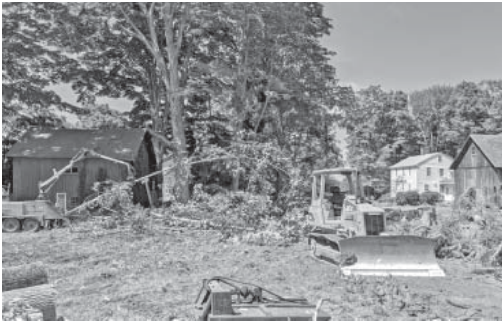
On Monday, crews were clearing land at 13 Church Street ahead of construction on the first building in Toomey's Crossing – a mixed-use development in the town center. Construction will begin in the next few weeks, with plans for the building to be finished by Thanksgiving.
