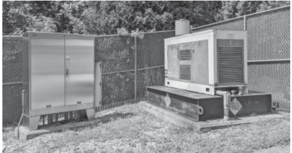
This generator at the pump station on Church Street will be replaced as part of a $7.6 million sewer upgrade project proposed for the town.
