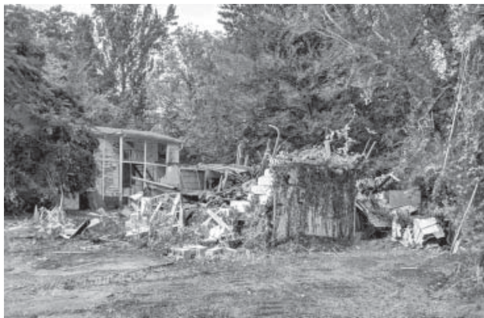
Demolition of some of the buildings on the former Elmcrest property started earlier this month.
