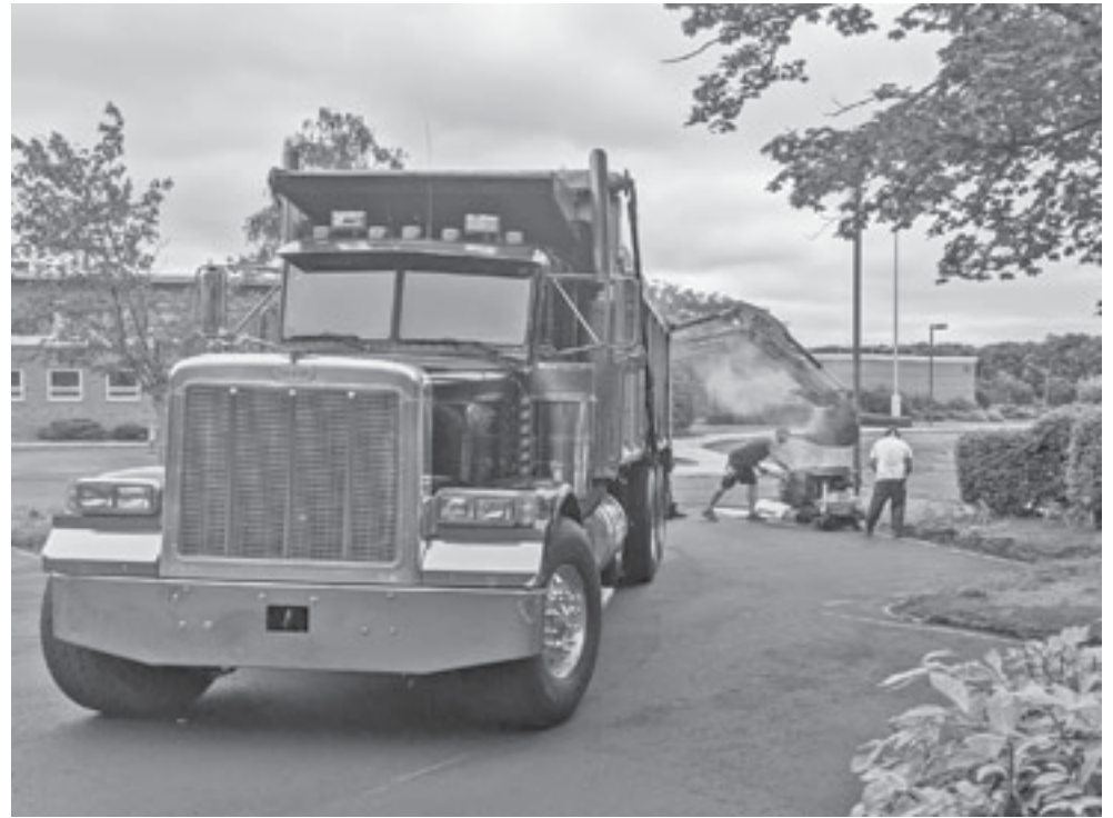
A crew pours asphalt at Gilead Hill School on Tuesday. The paving project, which is one of three moving forward in town this summer in addition to roadwork, should be done by the end of the week.
