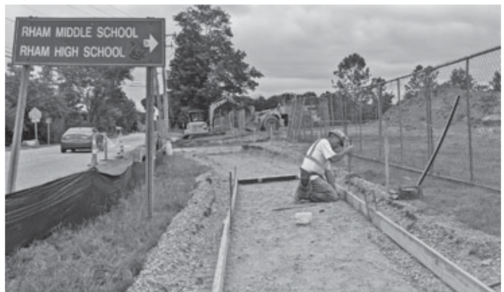
On Tuesday, a construction worker at RHAM works on a sidewalk while another worker in an excavator does some digging in the distance.
