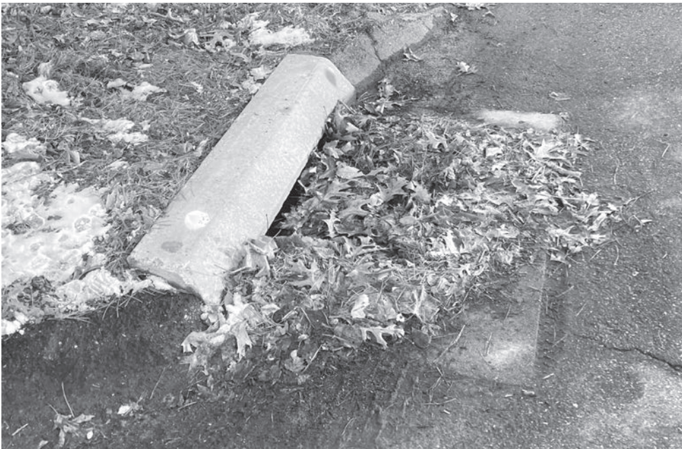
Clear Those Basins... This catch-basin or storm drain on a street near Lake Potopaug is almost completely clogged by leaves that can lead to flooding and algae growth. The Lake-Smart Committee said it is important for residents to remove leaves that can be blown into the streets and clog the drains. Leaves that enter town waterways add to the phosphates of the lake and contribute to the growth of algae, the committee said. Marty Podskoch photo.
