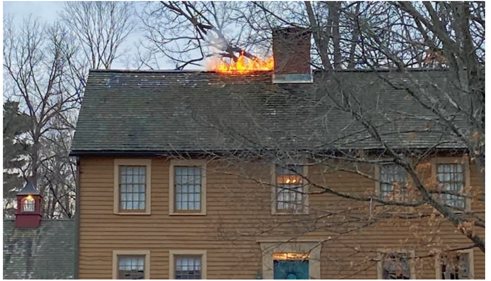
On Dec. 19, fire crews from both Portland and Middletown doused a small-but-serious fire on Indian Hill Avenue. Occupants were home, managing to escape with no reported injuries.
