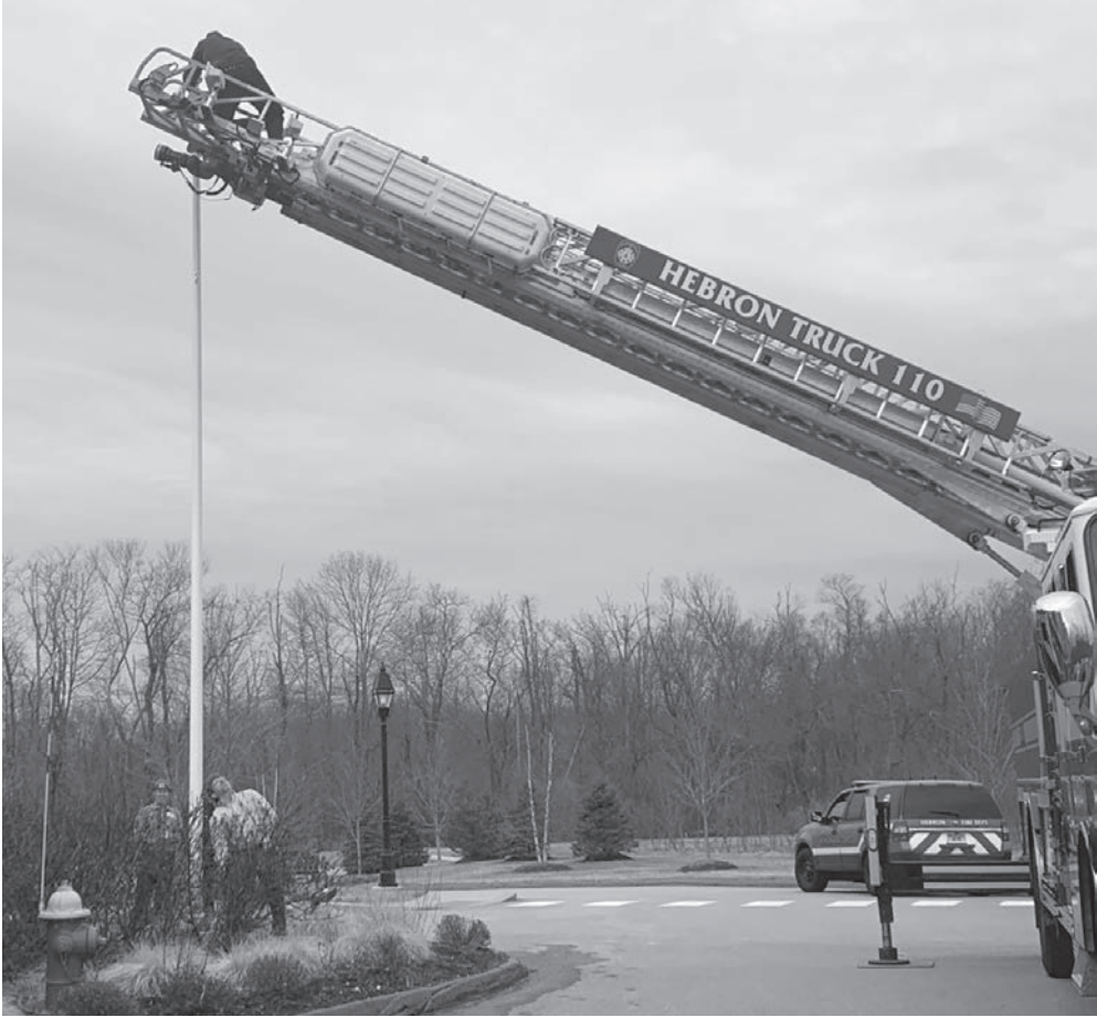
Fixing the Flagpole... Pictured is some ladder-truck training as the Hebron Fire Department helps to repair the Colebrook Village flagpole. The senior living facility offered thanks to Hebron Fire Department and EMS.
