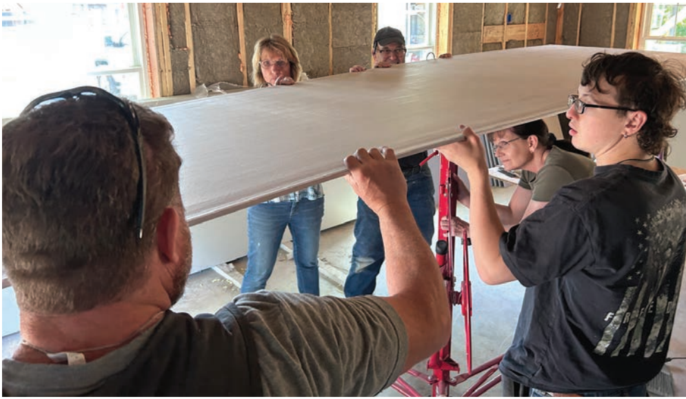
Habitat for Humanity Build... Eight members of Christ Episcopal Church, Middle Haddam, worked at a Habitat for Humanity site in East Hampton on May 20. The group helped hang sheet rock in what will be a four bedroom house located on Route 66. Habitat for Humanity is a nonprofit dedicated to helping individuals to obtain decent, affordable housing, for themselves and their families.
