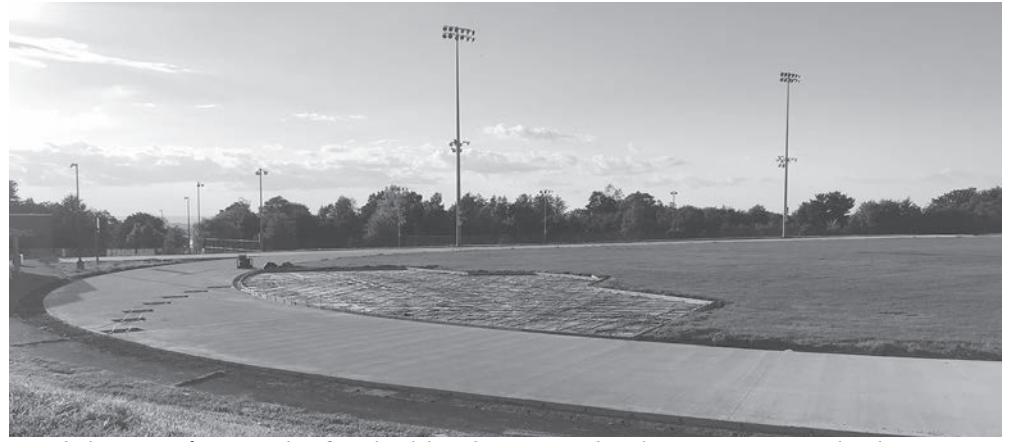
While it won't quite be finished by the time school starts next week, the revamp of the PHS track is well underway. The new-look track is expected to be complete by early October.
