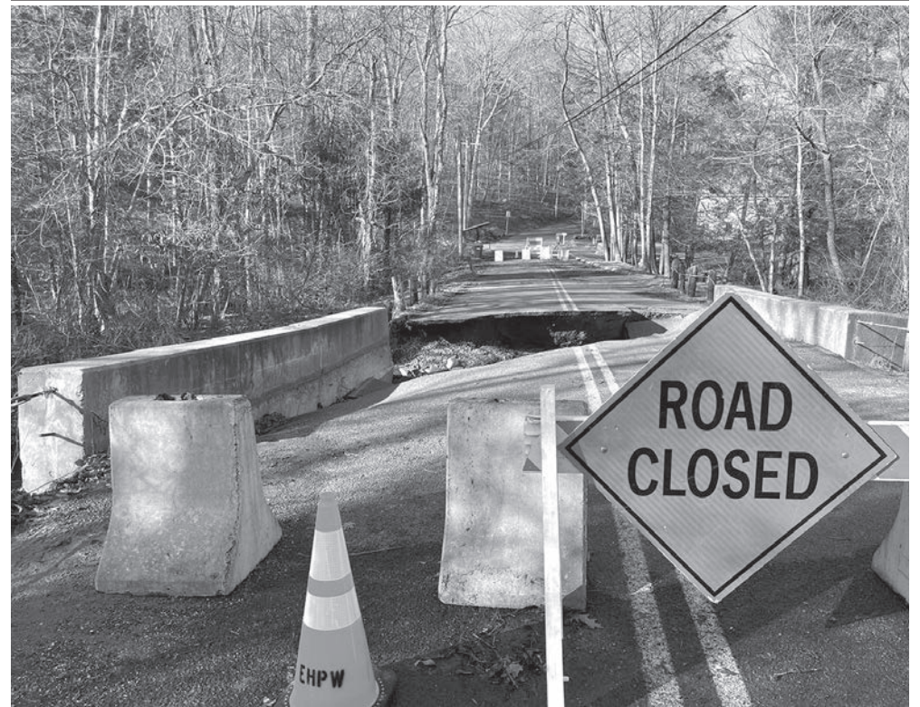
A culvert on Wopowog Road in East Hampton collapses for the third time due to large amounts of precipitation. The item has been slated to be redone for years but has yet to be a top priority.
