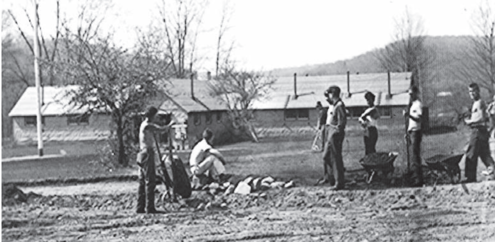
CCC Camp Stuart enrollees are shown working on their camp road and pathways in East Hampton. The camp was in existence from 1935-37. Photo by Chatham Historical Society.
