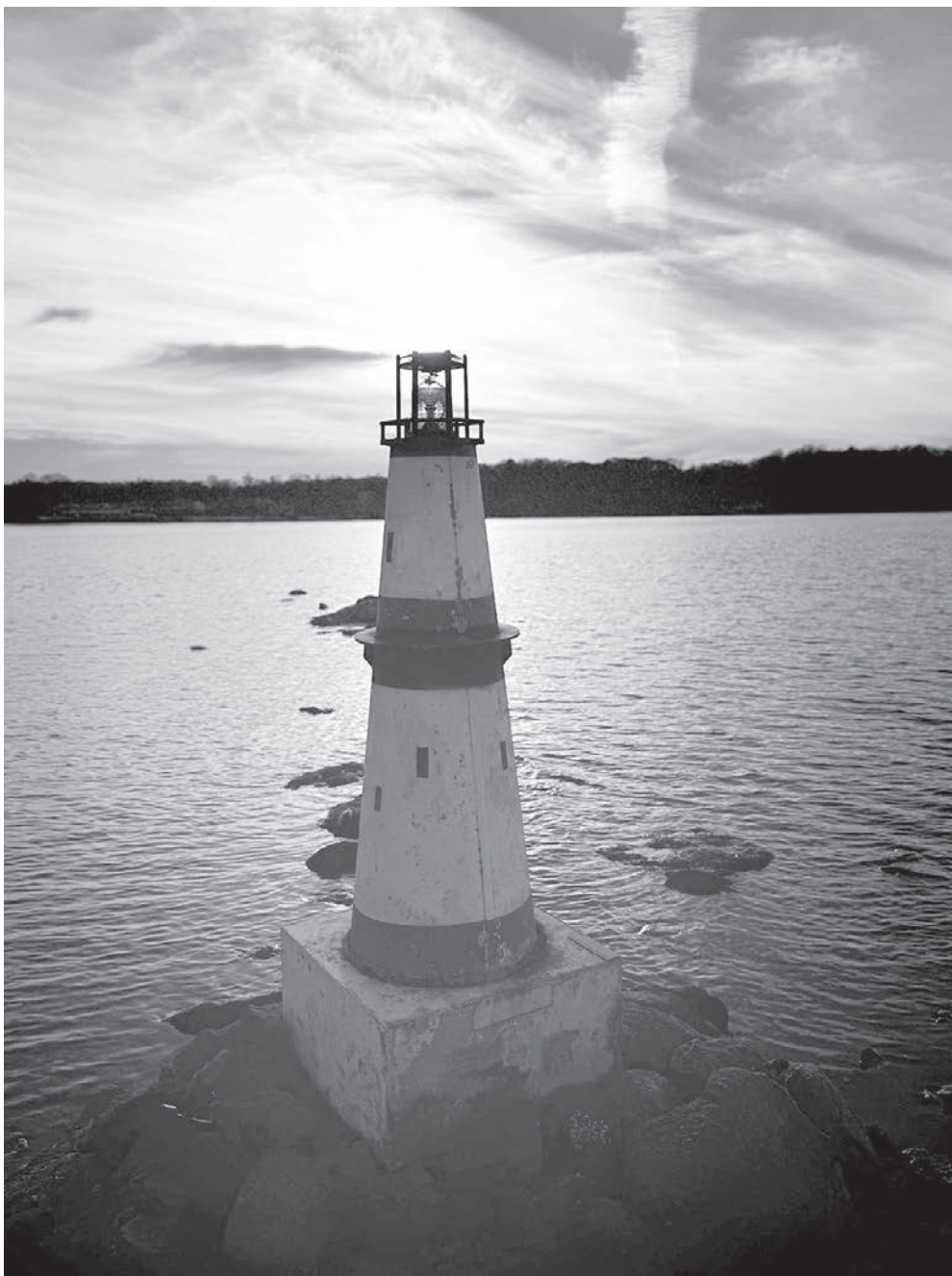
After years of looking at a crooked lighthouse without a working light, Cole and Dalton Peszynski researched the history to find the current owners. When granted permission, the two set out to fix it to ensure boaters' safety near the rocky island. Photo by Cole Peszynski.
