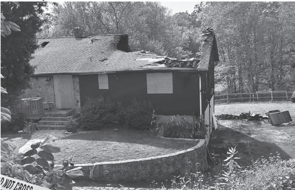
A fire Sunday left a home on Isleib Road heavily damaged. The residence has been deemed a total loss.
